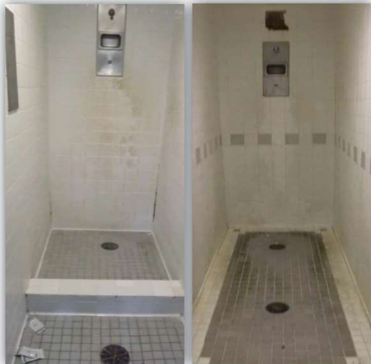
Figure 3. Moldy, mildewed shower stalls observed by OIG at TLF on November 16, 2016 Source: OIG
