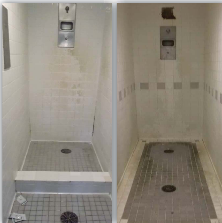
Figure 3. Moldy, mildewed shower stalls observed by OIG at TLF on November 16, 2016 Source: OIG
